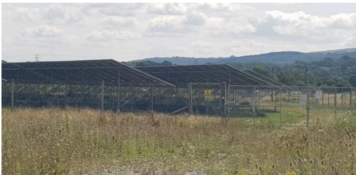
Figure 2-14. Typical Fence and CCTV System at a UK PV Facility
