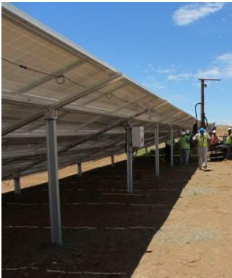
Figure 2-8. Example of fixed tilt solar panels on H-style steel piles
